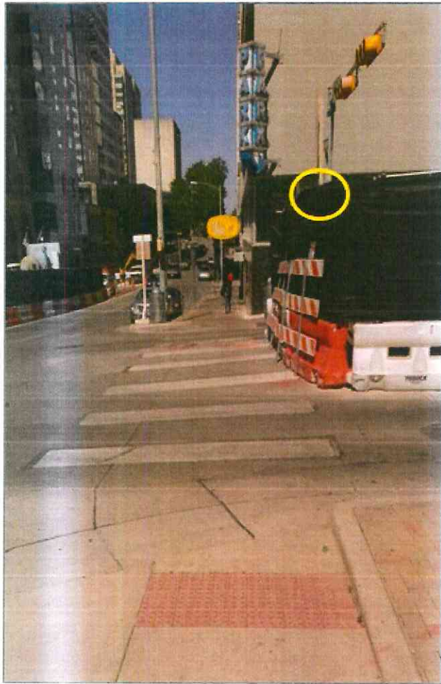
Figure 6. Work zone devices and materials can obscure pedestrian signals can make it difficult for pedestrians and right-turning vehicles to see each other (Source: FHWA)
