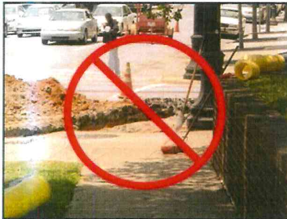
Figure 1. Open holes and trenches on or near pedestrian routes must be protected (Source: TTI)
