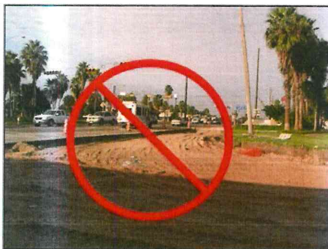
Figure 4. Sidewalks should not lead directly into unprotected work spaces (source: TTI)
