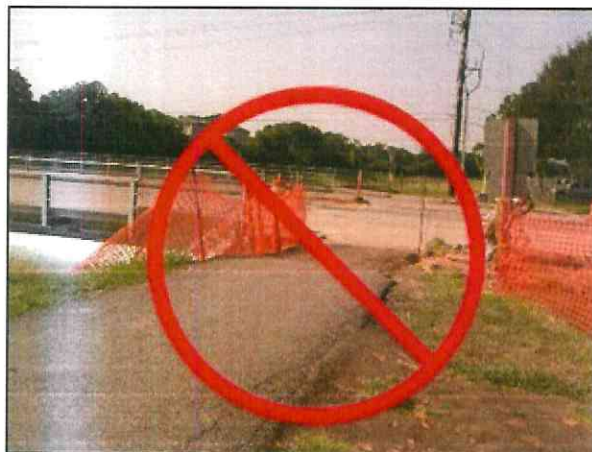
Figure 2. Mesh fencing is not sufficient to protect a pedestrian from falling into a trench or hole (Source: TTI)
